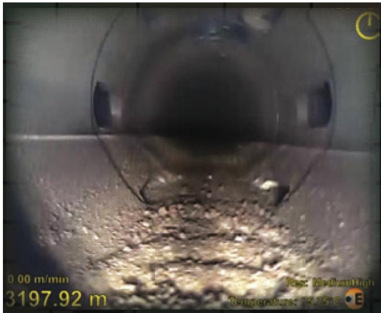
FIGURE 10 – SOLIDS DUNE/BED MIGRATION ACCUMULATION NEAR THE BASE OF THE WELLBORE’S CURVE SECTION
